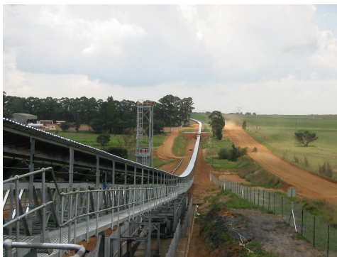
Figure 3: Ingwe Overland Conveyor System in South Africa
